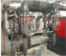
St. Priest, France Geothermal Heat Pump
