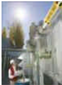
Mountain View, CA Landfill Gas Generation
