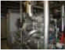
United Kingdom Ammonia Chillers
