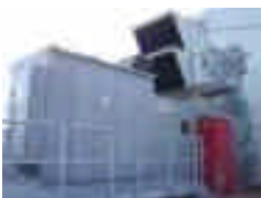
Raritan, NJ Gas Turbine
